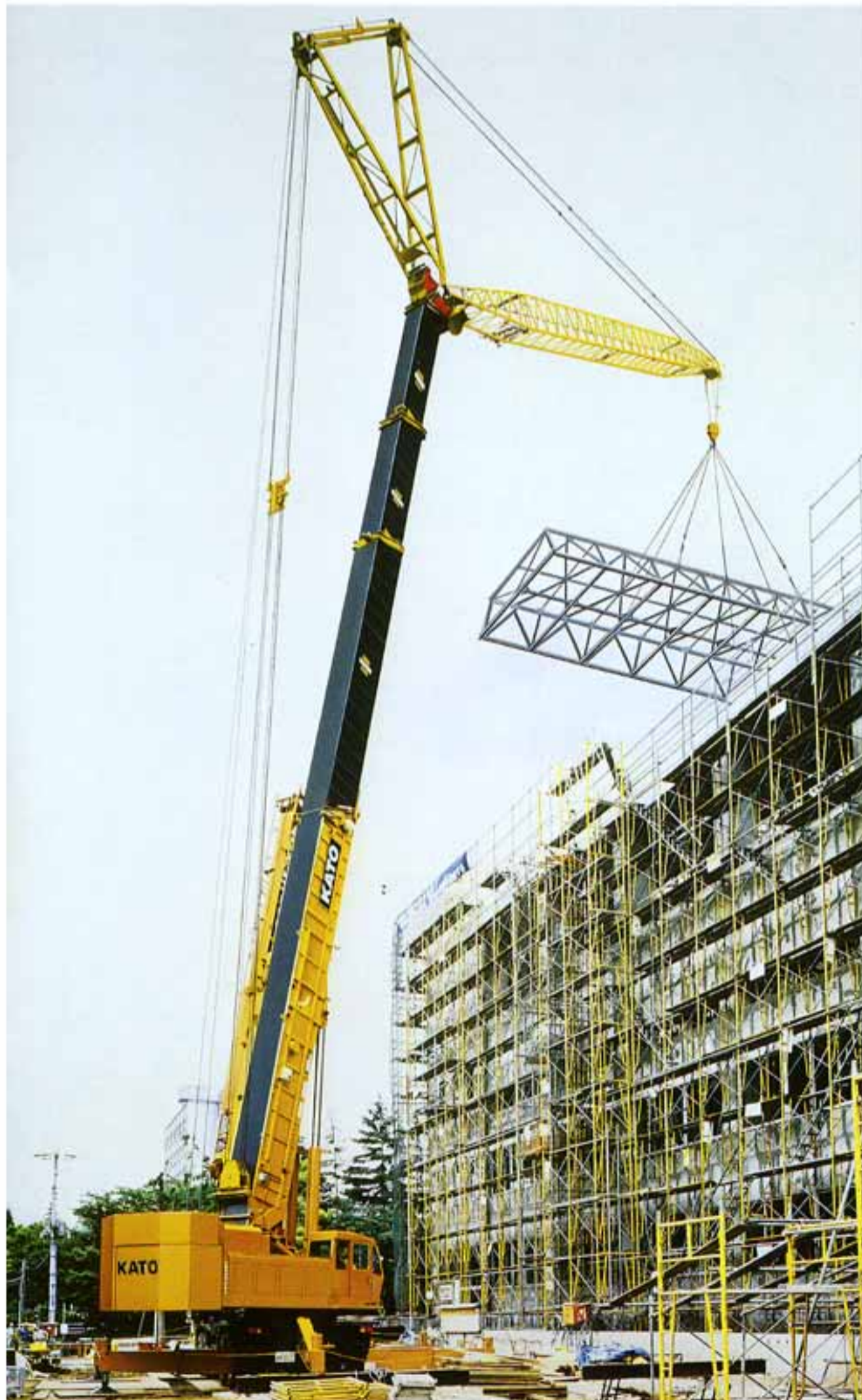
The installation of extra large load using the main boom and heavy lift jib. (Domestic model)
