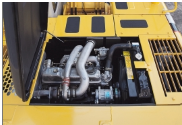
●Engine room (Equipped with air conditioner-option)
